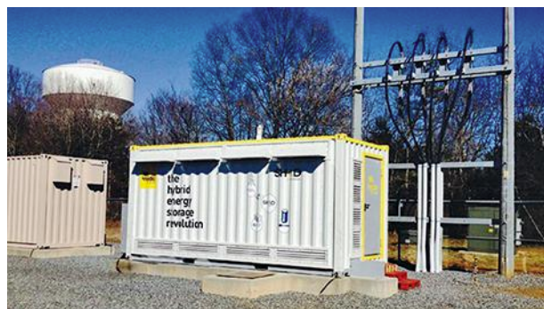
1. This hybrid battery-supercapacitor energy storage system was deployed at a distribution substation in Gaston County, N.C. (Courtesy of Duke Energy)
